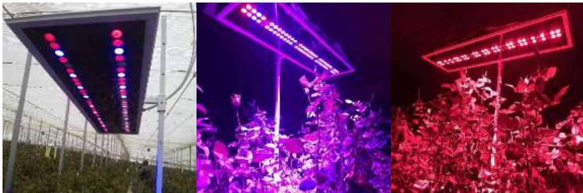
Fig. 1. LED lamps installed in the greenhouse.
